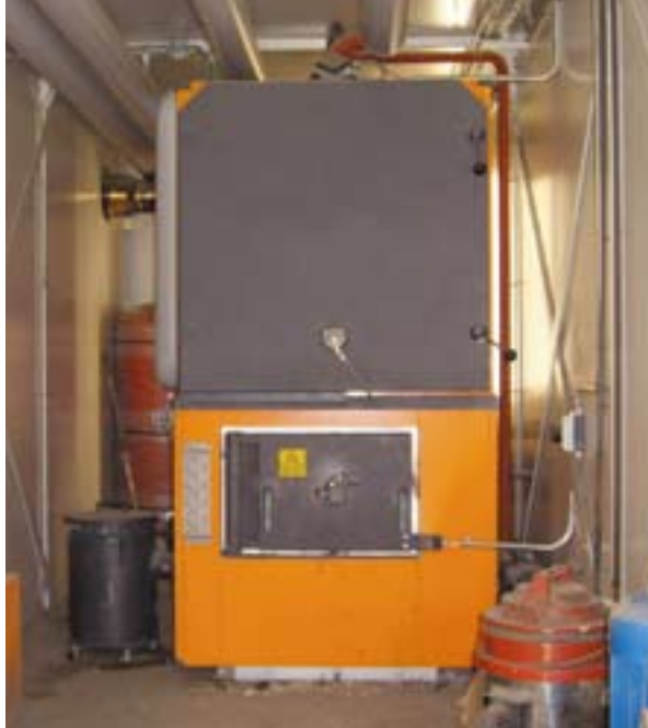
Medium size boilers can be used to heat schools, hospitals, public buildings, groups of apartments, small district heating networks, etc.
